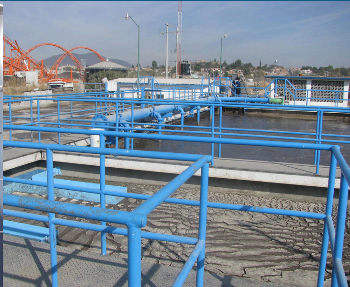
SANITATION: Santa Rosa Jáuregui Wastewater Treatment Plant - Santa Rosa Jáuregui, Municipality of Querétaro, Querétaro.
